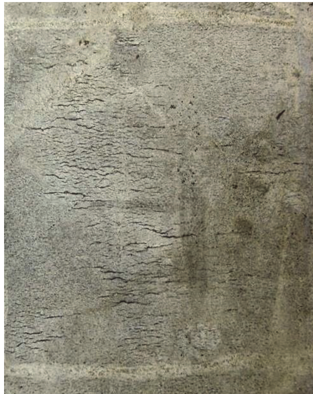
Figure 1—External Surface of Pipe Sample with Sulfide Stress Cracking
